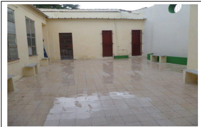
This photo was just taken – January 2012 and sent by email. It shows a mostly completed section of the Guanabacoa Presbyterian Church, in Guanabacoa, Cuba.
